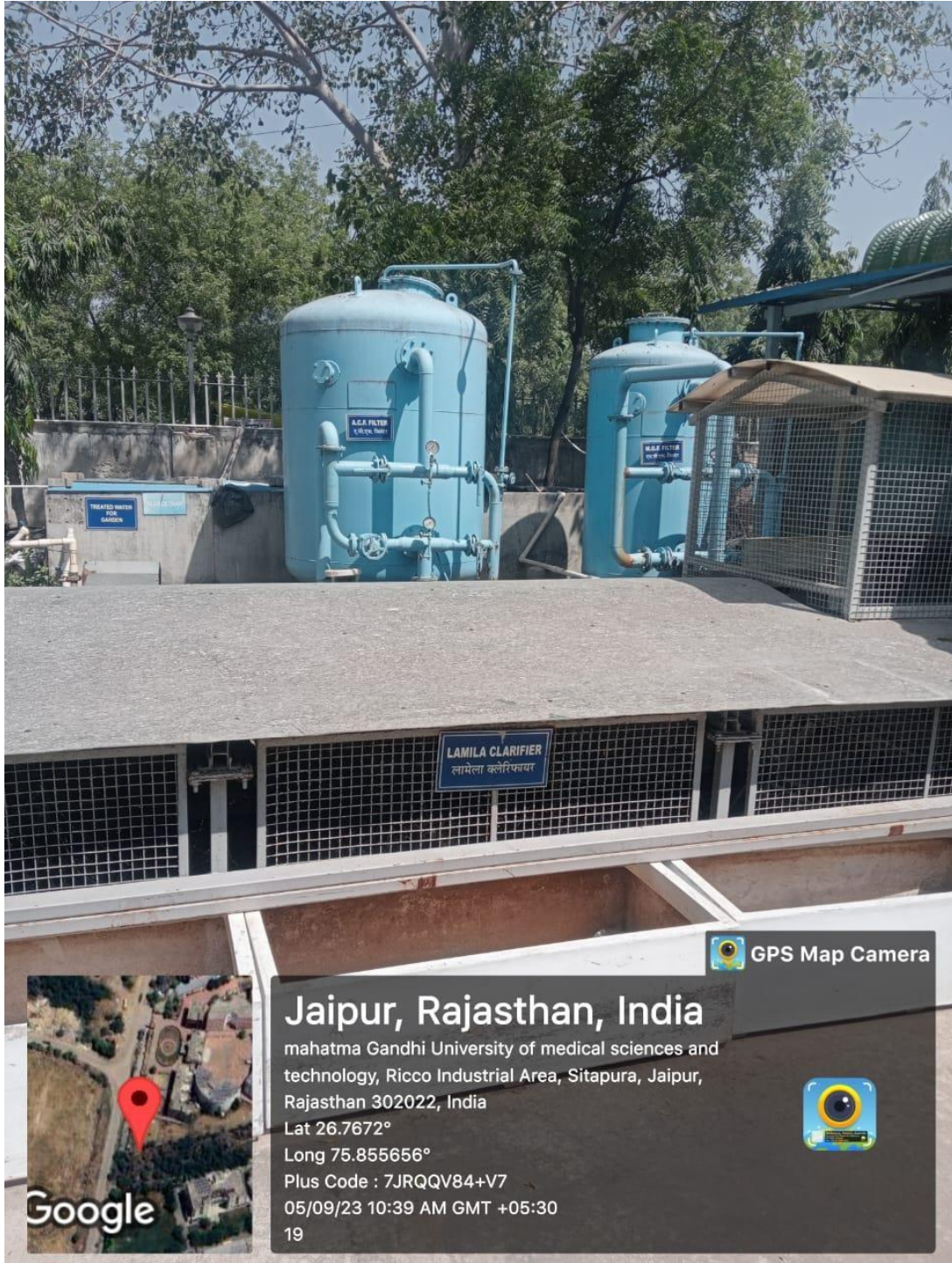
FILTERS & LAMILA CLARIFIER IN SEWAGE TREATMENT PLANT
