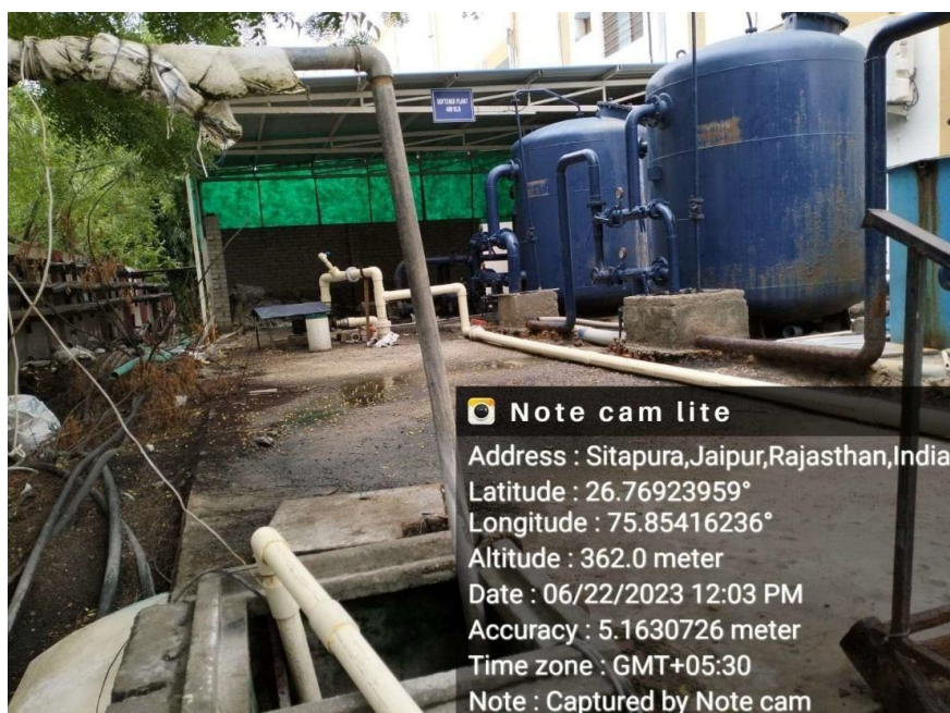
Fig-8: Photographs of RO Plant
